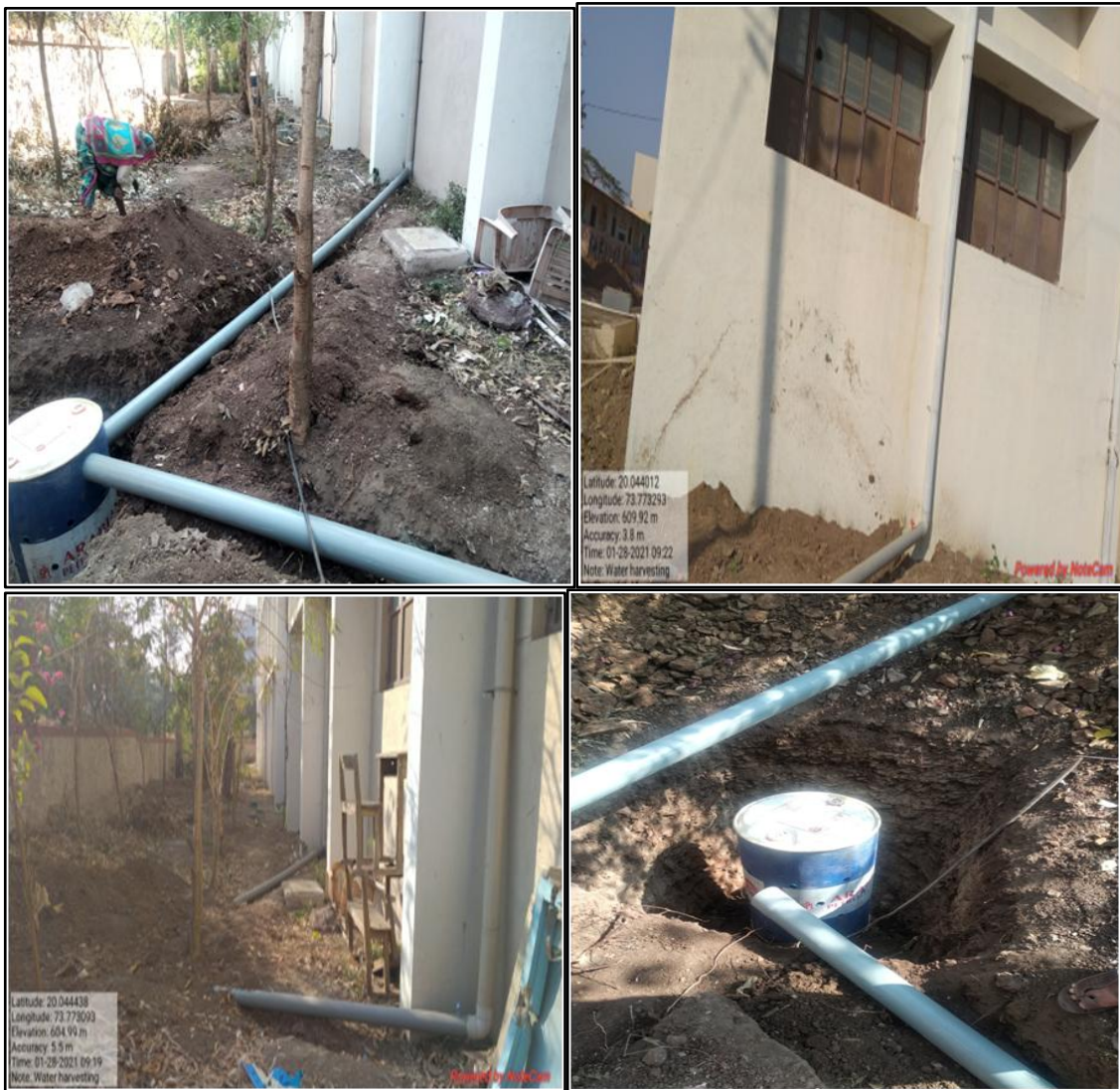
Fig : Rainwater harvesting and collection system in the college campus
